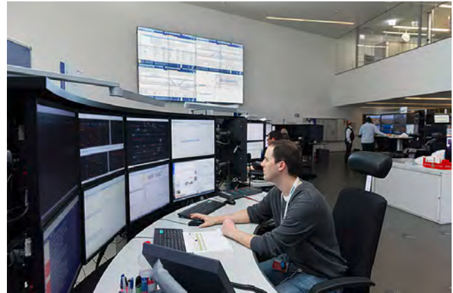
Control room with WinCC OA
